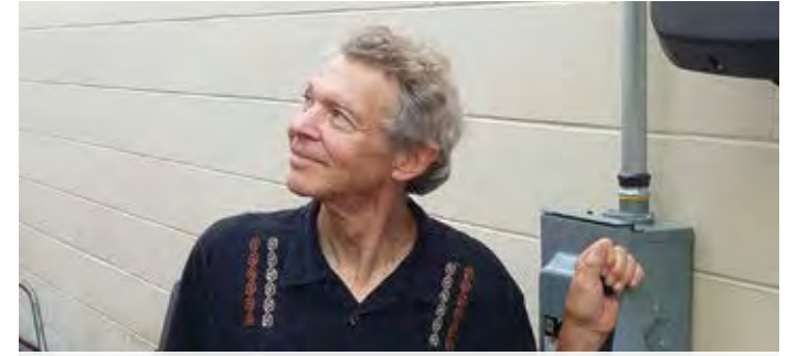
Don Wichert flips the switch to activate the solar system on the roof at the Willy Street Co-op.
